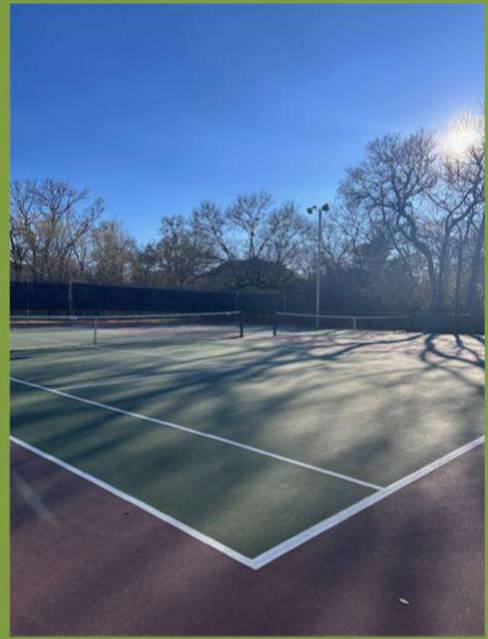
Tennis Court surface installed in 2014. We have passed the ten year life expectancy.
